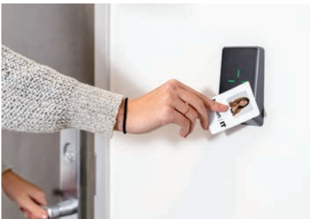
Secure Access Control
