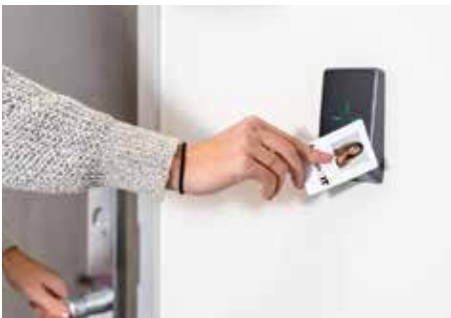
Secure Access Control
